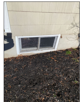
Poor foundation clearance
