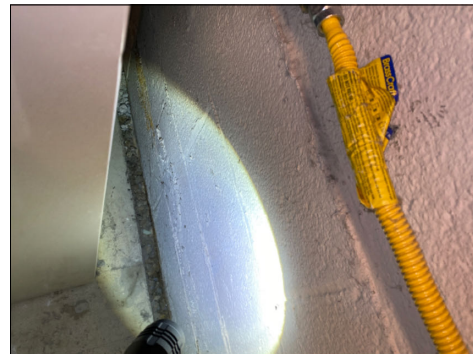
Water staining / efflorescence
