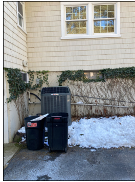
Vegetation on walls
