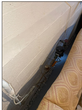
Main water shutoff
