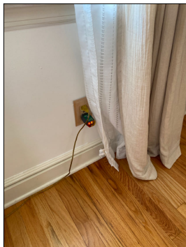
Incorrectly wired receptacle, #1
