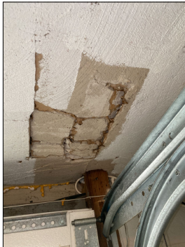
Sheetrock not continuous
