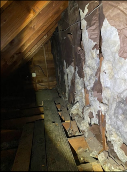
Incorrectly installed insulation
