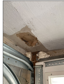
Sheetrock not continuous
