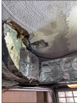
Sheetrock not continuous
