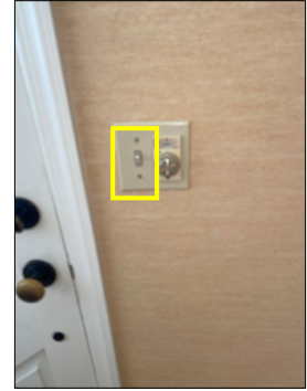
Inoperative / unknown fixture control
