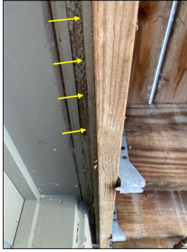
Ledger board over siding
