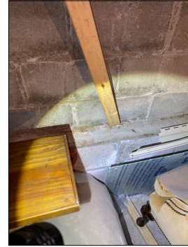
Water staining / efflorescence
