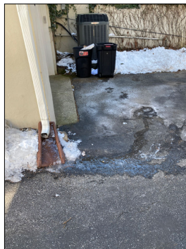
Discharge too close to foundation
