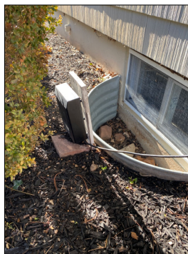
Low voltage light board
