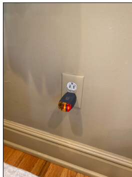
Incorrectly wired receptacle, #2
