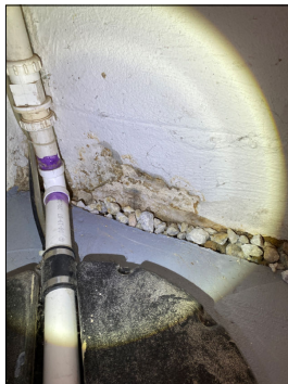
Water staining / efflorescence
