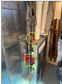
Gas and Electric Shutoff
